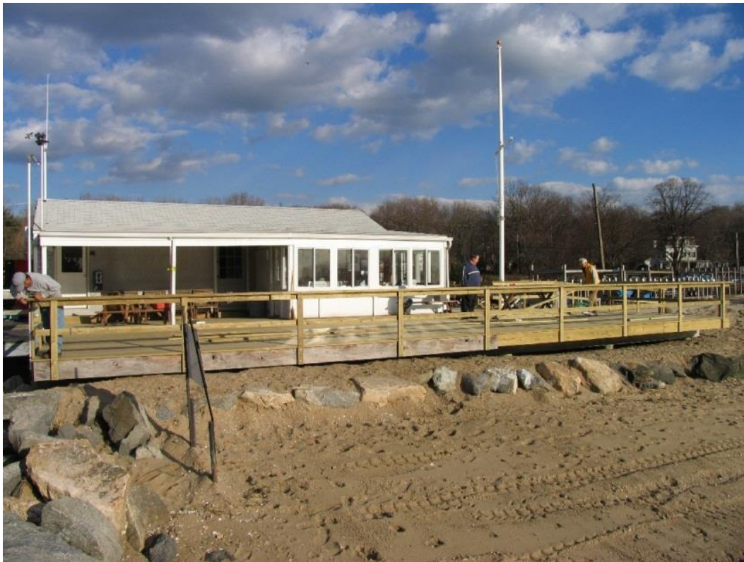
Prior to the storm the club had a beautiful deck that was increased in size and finished in 2004.
